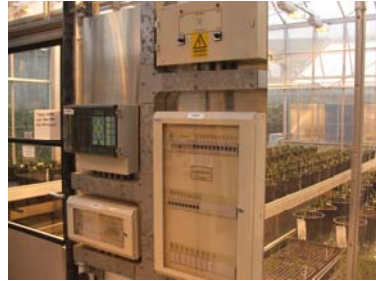
Typical Glasshouse compartment with adjacent Envirocon controller.
