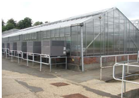
G28. Polycarbonate clad, air conditioned.
