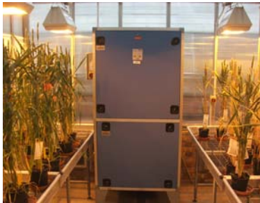
Air conditioned compartment from G31. Note polycarbonate cladding and air conditioning unit
